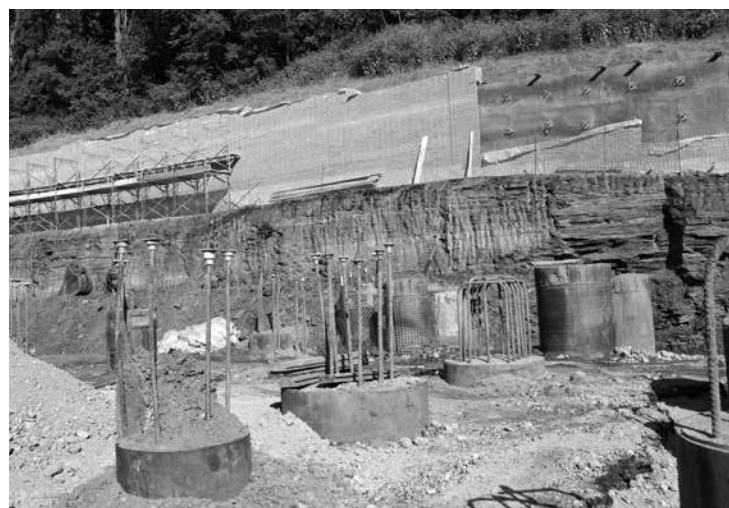
Caisson rebar being cleaned and ready for grade beam installation. In the background the Soil Nail wall is being faced with brick to match the PEC and the new Salk Addition.
